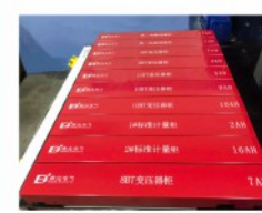
机柜眉头 Cabinet sign
